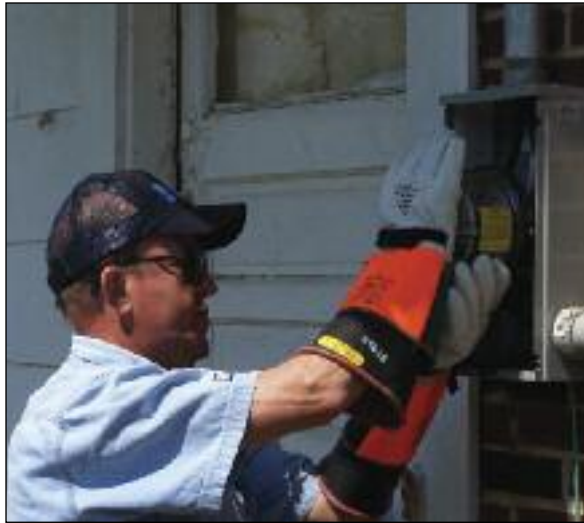
Morris Carothers installs a turtle meter. It transmits a reading approximately every 27 hours.
